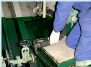
Illegal pipe – sludge pump to overboard
